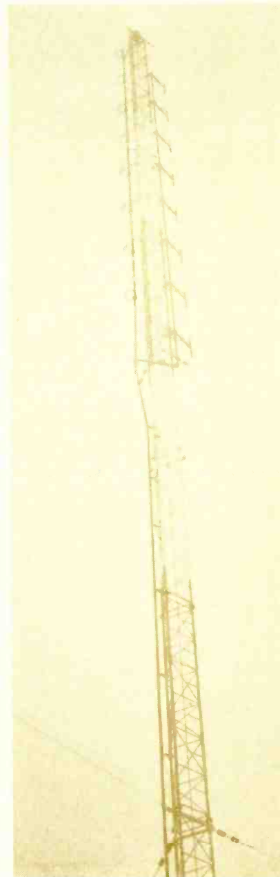
The FM antennas shown installed on the new tower.
